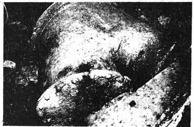
D Y-junction in turbine feed pipe at Lower Wireworks site; right-hand branch feeds turbine, left-hand branch blanked off.
